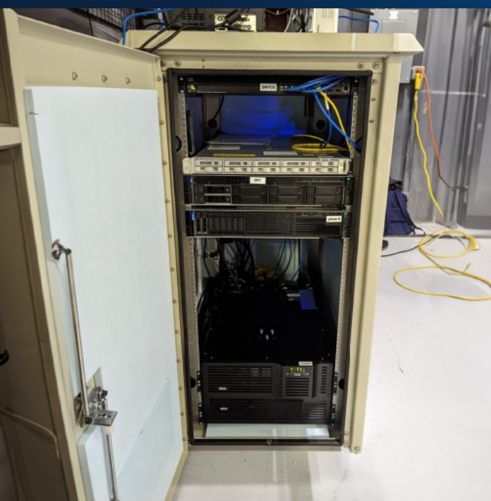
Figure 1: Single rack carrying 4G/5G Core, baseband, power supply, and distribution switch.
